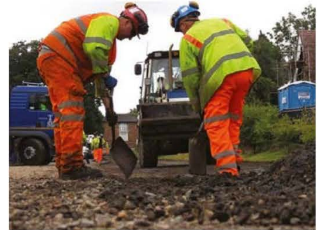
Dressing a road surface and, right, a highways team performs essential road preparation
